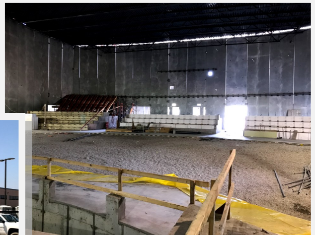
Auditorium Seat Risers
