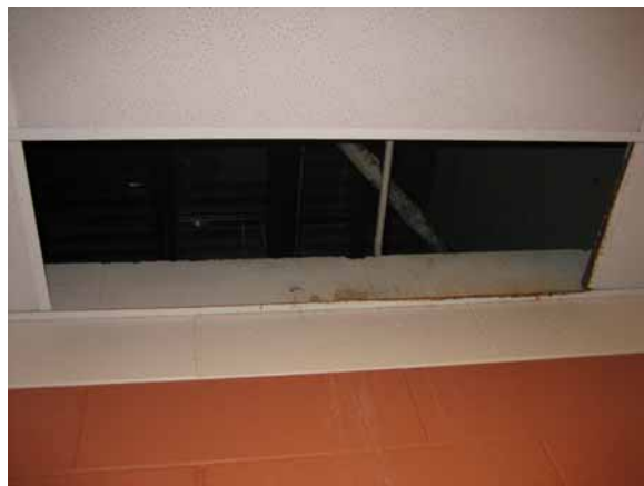
2.3 Interior leaks from roof above
