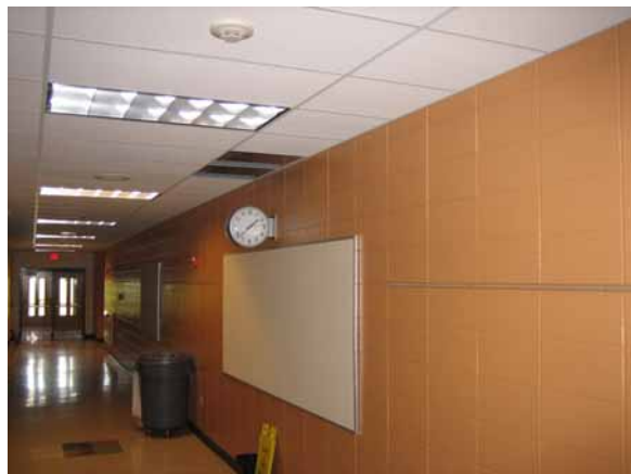
2.3 Interior leaks from roof above
