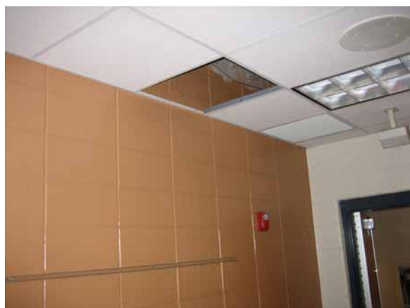
2.3 Interior leaks from roof above
