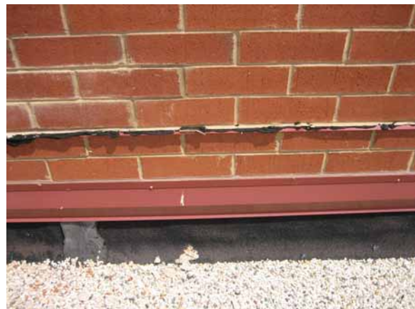
2.3 Flexible membrane flashing failure at gym wall
