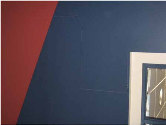
4.9 Cracks in library walls
